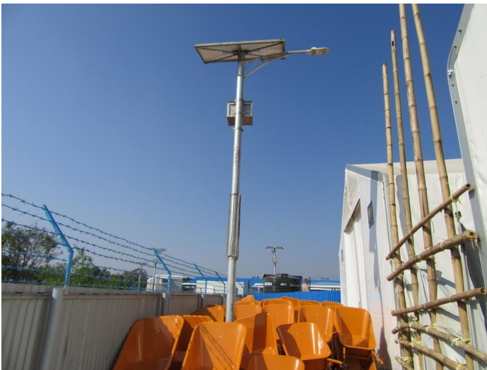
Solar light installed at IOM logistic base. ©IOM 2017
